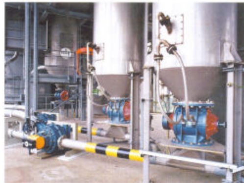
Product feed from silo via rotary valve.
