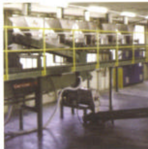
Five weigh feeders and a continuous mixer, feed a calender roll for PVC floor coverings.
